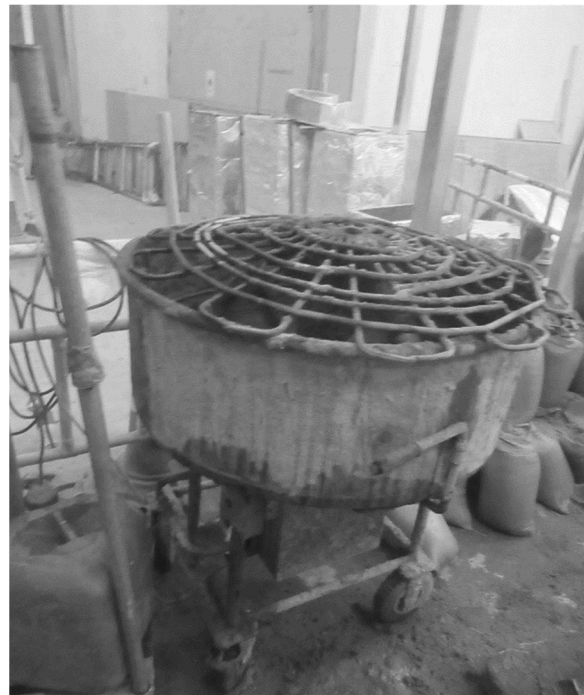
Figure 7. Wet cement sand mixing for building a brick wall at a renovation site.
